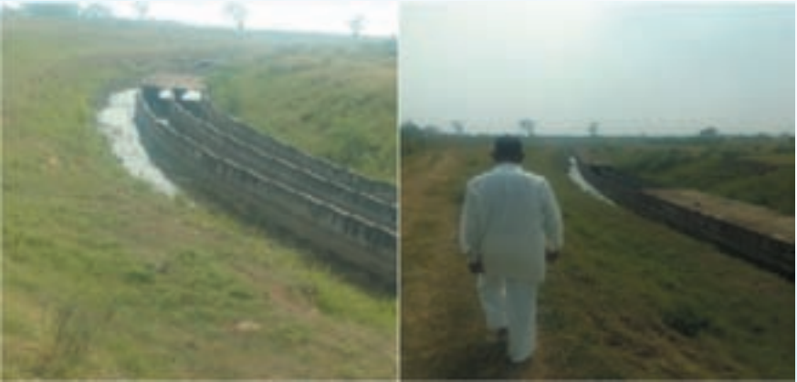
Spillage of water between Chainage 760 and Chainage 782 during Joint Physical Verification
