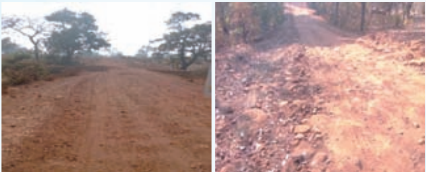
A view of incomplete work at km chainage 1,200 and 2,100 of Anarad to Nihaldevi road as on January 2017 due to delay in proposal for acquisition of forest land
